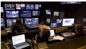
Master Control Room
